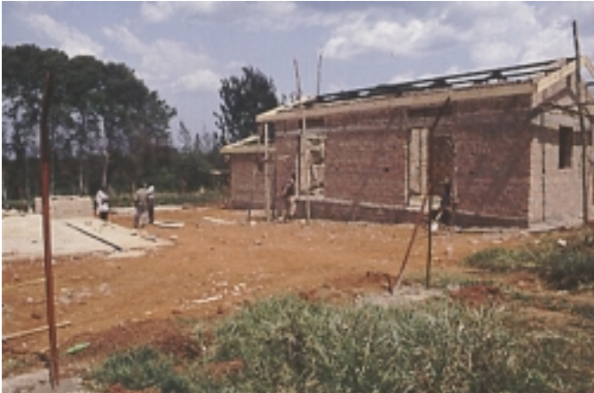
◀ The site of the Uganda Tree Biotechnology Project at Kifu in February 2002.
